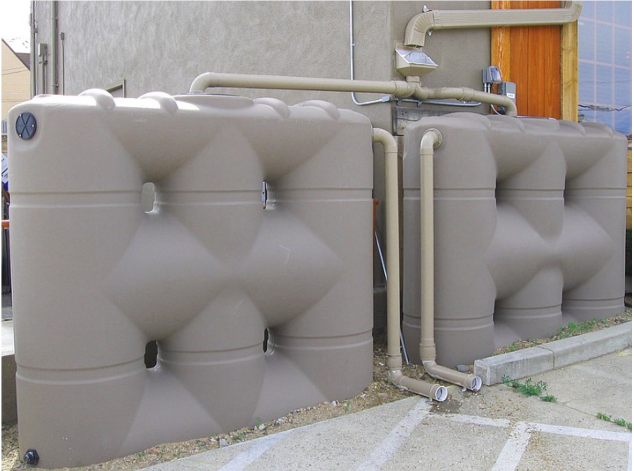
Large rain tanks at Prescott Station Restaurant. (Fred Oswald/courtesy)
