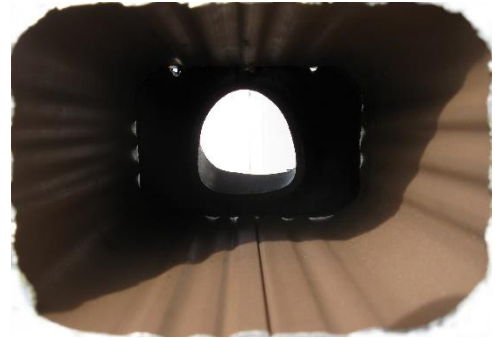
Fig 3 – Rubber diverter in downspout that blocks \frac{3}{4} of its area. Note small opening for passing water.
