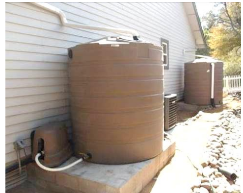
Fig 9 – Twin 650-gallon rainwater tanks beside Prescott home.
