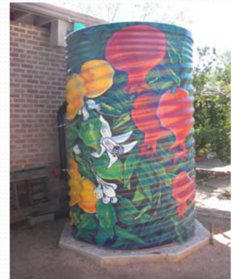
Rainwater harvesting tank. Photo: Christina Bickelmann
