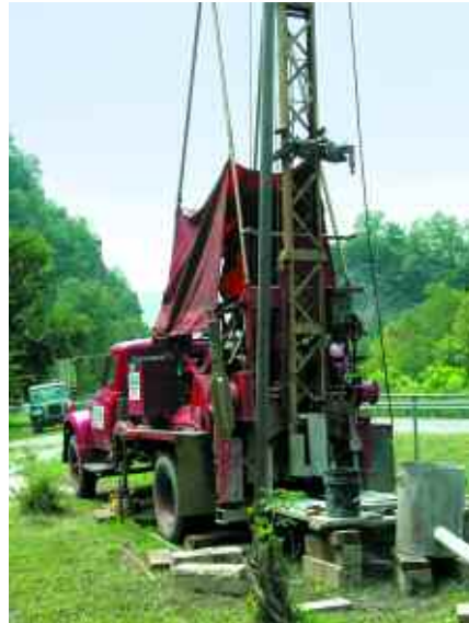
Truck-mounted groundwater wells have made water extraction in previously inaccessible locations possible.
