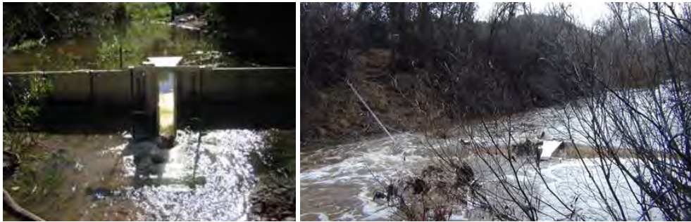
Walnut Creek Flume after installation, looking upstream (October, 2014) and after storm damage, looking upstream (January, 2015).
